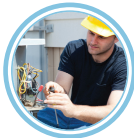
HVAC Service and Maintenance
